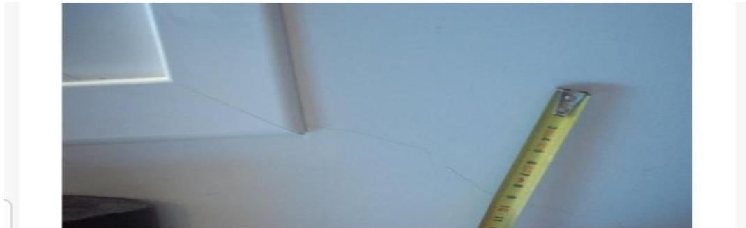
Fig. 4: shows cracks at the bottom of the window
