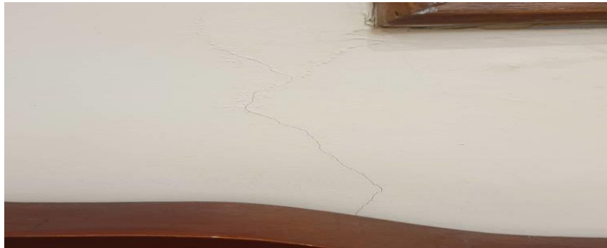
Fig. 1: shows cracks at the bottom of the window
