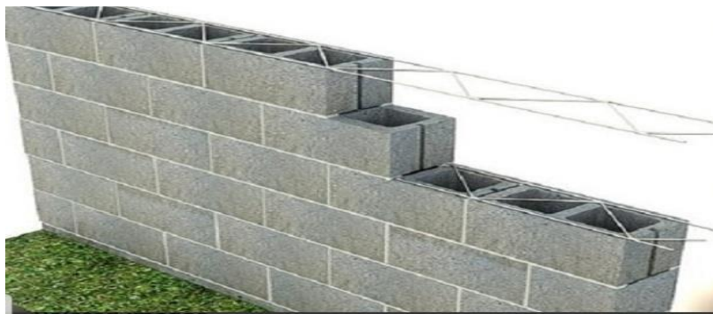
Fig. 5: shows the method of supporting the walls with an iron grid of diameter ( \varnothing 10mm)
