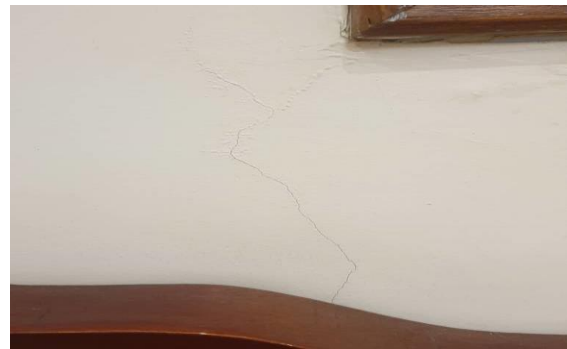
Fig. 1: shows cracks at the bottom of the window
