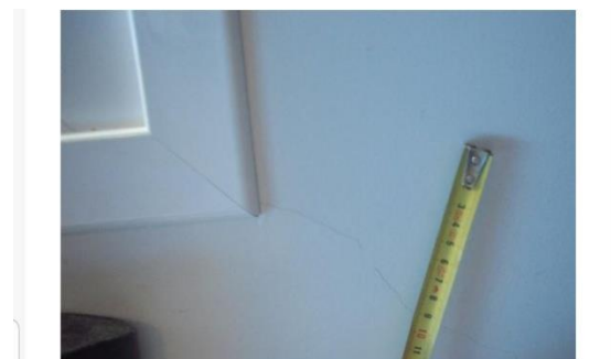
Fig. 4: shows cracks at the bottom of the window
