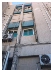
Fig. (7): Severe deterioration of all columns of the northern facade facing the sea
