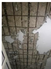
Fig. (11): The concrete cover of the slab on the third floor fell as a result of corroded steel reinforcement
