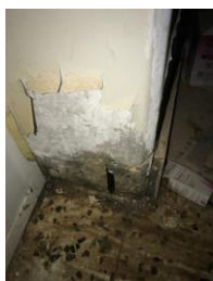
Fig. (14): Corrosion of reinforcing steel and spalling of the concrete cover which is less than 1 cm
