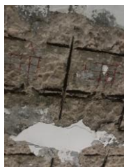
Fig. (12): Corrosion of the reinforcement steel and the collapse of the concrete cover of the slab on the second floor
