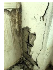
Fig. (10): Spread of corrosion of reinforcement steel for the same column on the third floor.
