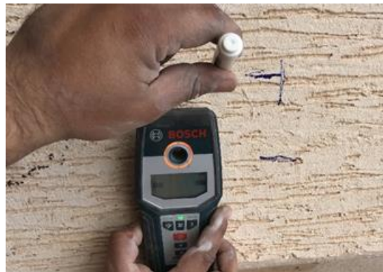
Fig. (15): Using a cover meter to indicate the location of reinforcement before taking core
