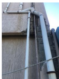
Fig. (13): Corrosion of steel due to leakage of sewer and sewage pipes
