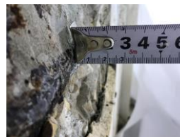
Fig. (5): The thickness of the concrete cover ranges from 1 cm to 2.5 cm for the columns
