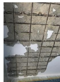
Fig. (6): The thickness of the concrete cover is less than 1 cm in the slabs
