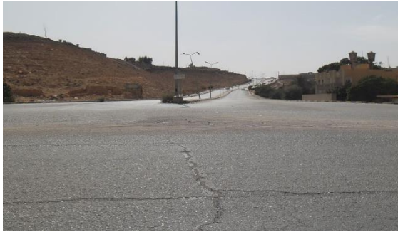
Fig. 2: Damages in the intersection
