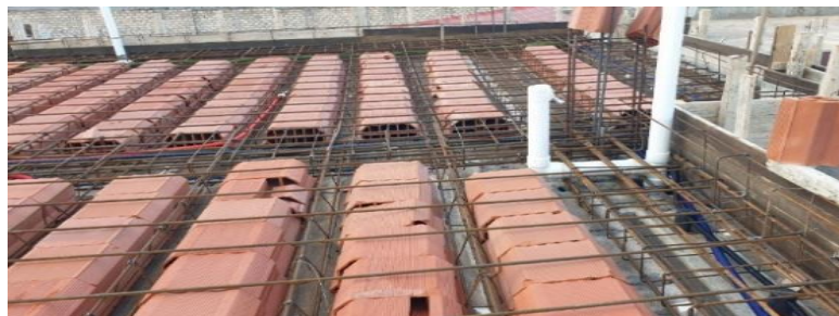
Figure 9 sewage pipes inside the beams
