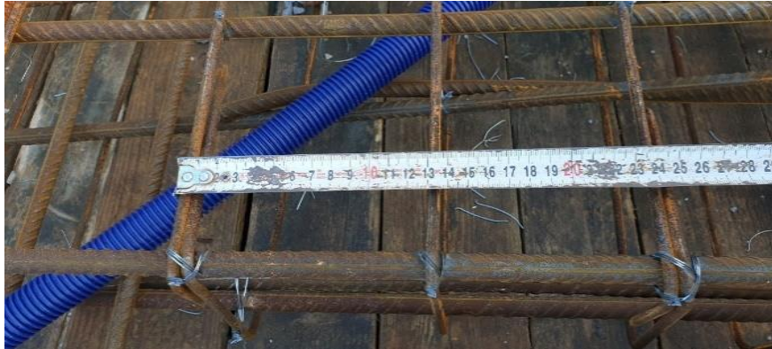
Figure 7 the spaces between the stirrups are uneven
