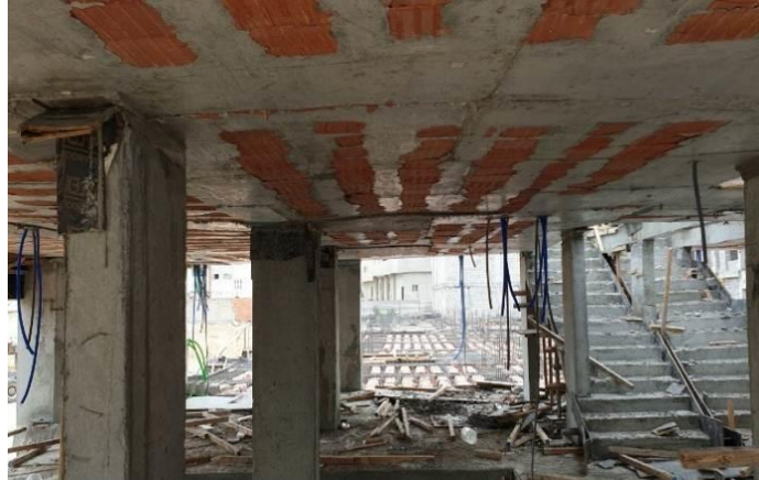
Figure 13 The deflection of the slab due to poor supports
