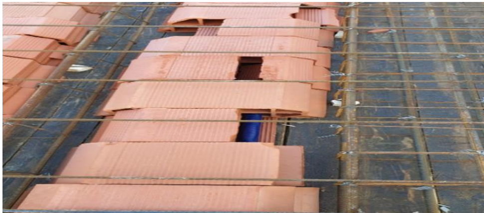
Figure 8 The Shape of broken bricks
