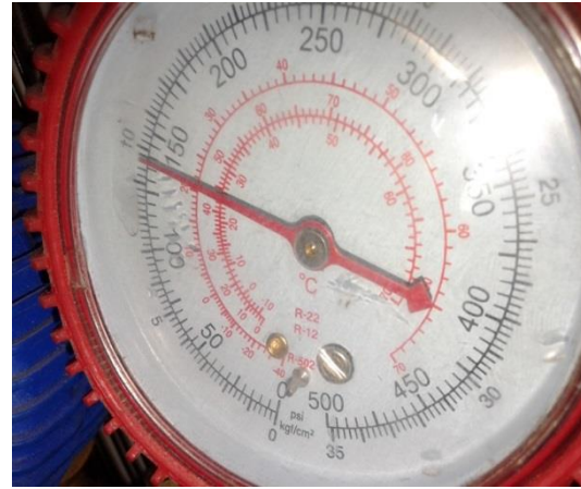
Figure (4) shows High pressure gauge.
